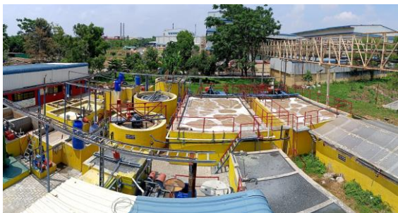
Hosur Effluent Treatment Plant – Zero Liquid Discharge
